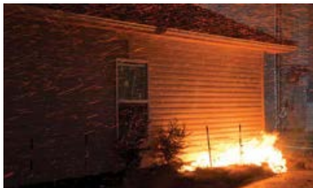
Flying embers are the most common source of home ignition during wildfires. Preparing homes for their impact is critical. Embers can ignite leaf litter in gutters and on roofs, as well as shrubs and mulch at the base of the house, as seen in this controlled ember shower experiment. Photo: Insurance Institute for Business & Home Safety
